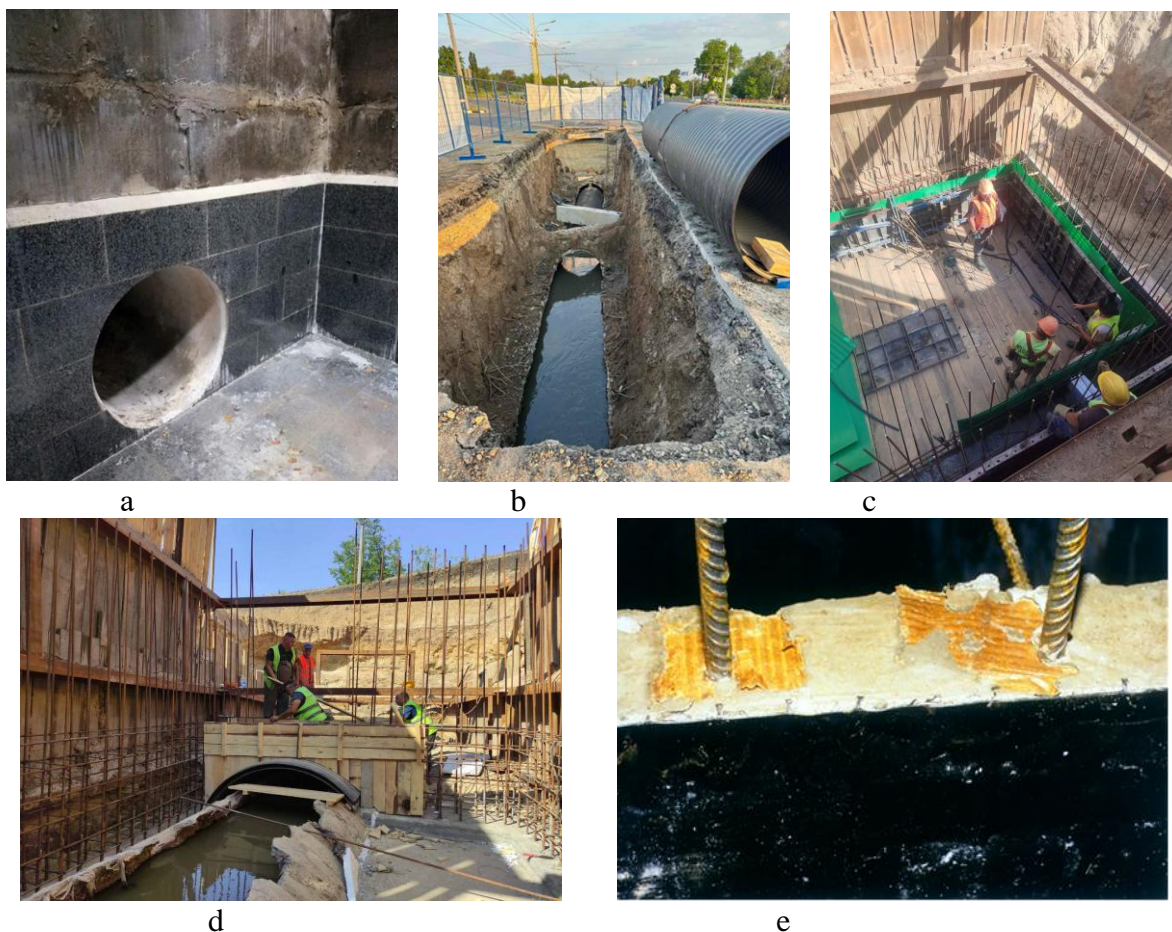
Fig. 3. Application of various modern materials for the rehabilitation of wastewater infrastructure facilities in the city of Kharkiv: a – Restored energy-dissipation chamber K-1 using porcelain stoneware tiles; b – Rehabilitation of a section of the sewer tunnel along Aerokosmichnyi Avenue (Kharkiv) using open-cut installation of 1500-mm CORSIS polyethylene pipes; c – Construction of an inspection shaft with wall lining using ribbed polyethylene panels; d – construction of the tunnel using a polyethylene vault insert; e – Rehabilitation of the inspection shaft using ribbed polyethylene; f – Lining of the inspection shaft using slag-cast panels; g – Laboratory investigation of polymer concrete at KhNUBA; h – Ceramic tile lining of the sewer manhole; i – Rehabilitation of the collector segment using profiled polyethylene lining; j – Collector rehabilitation via spiral-wound polyethylene lining
